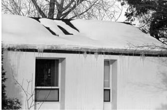
Photograph 1. A single-story house with an ice dam. The areas without snow are the points of heat loss.
