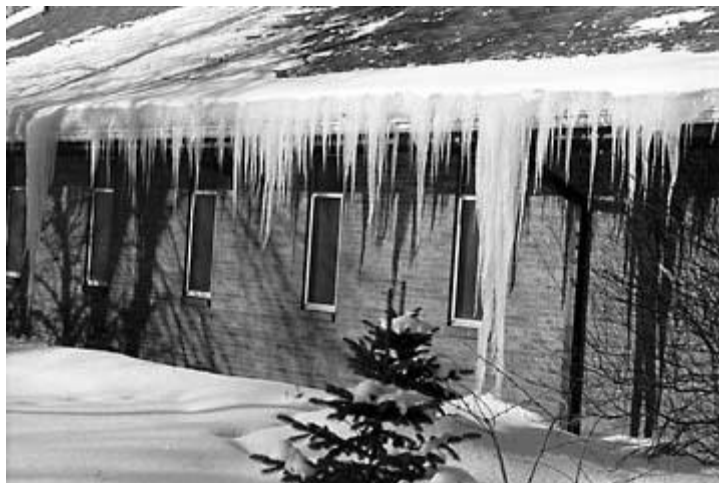
Photograph 2. The unusually high heat loss on this roof has caused both an ice dam and icicles.
